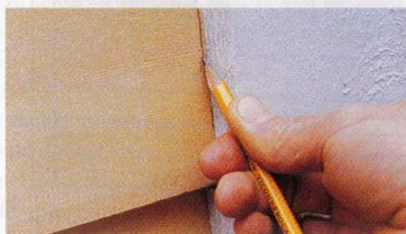
Scribe the end of a clapboard by drawing the side of a pencil along the edge of the trim board. Then trim the waste down to the scribed line with a low-angle block plane.
