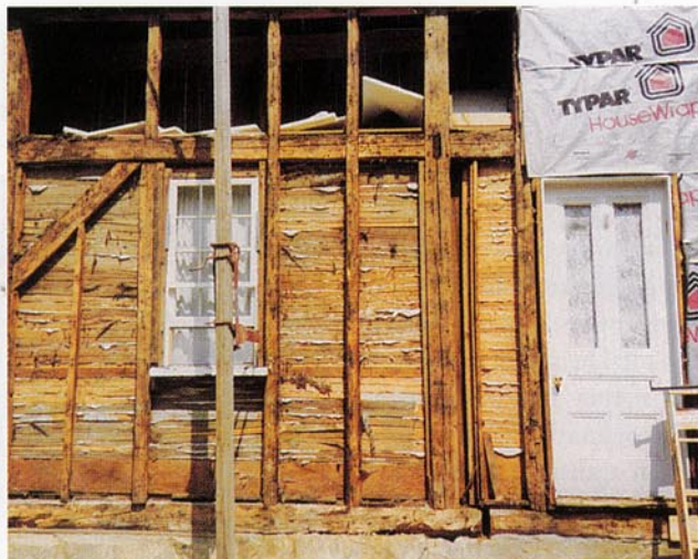
Removing later siding and original sheathing boards exposed the structural frame for inspection and wiring. Note the split-board lath and plaster.
